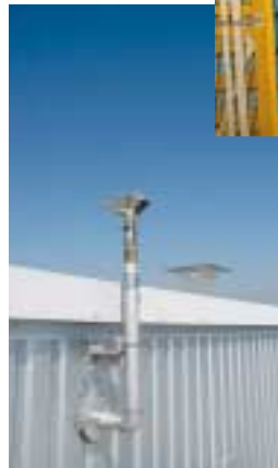
Air-conditioning cost is reduced by means of a roof sprinkling system, external insulation and natural air circulation. Natural light is also used to reduce lighting cost in this highly economical facility structure
