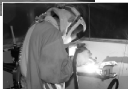
Where extra skill and precision are needed, the welding is done manually by expert welders
