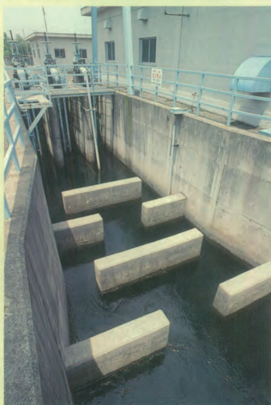
A water supply mixing trough
