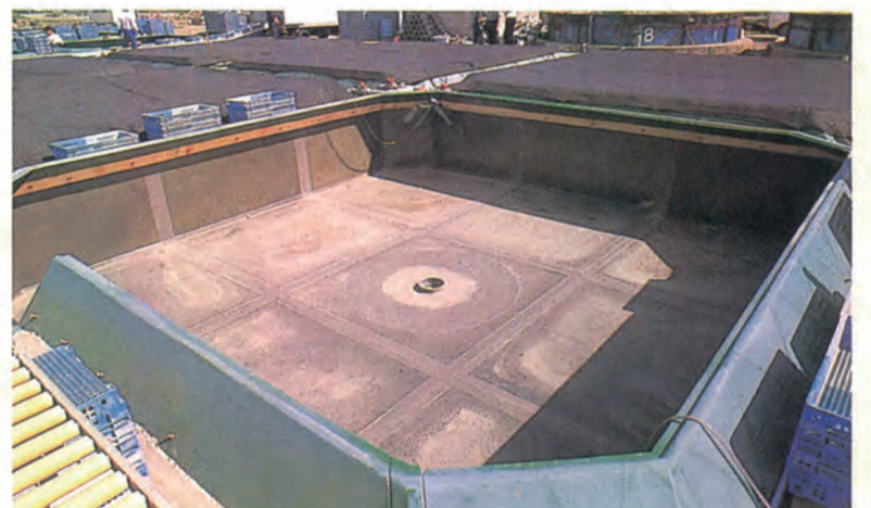
A square type tank (6m x 6m). A drain is located in the center.
