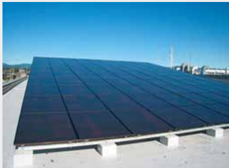
Solar generation system introduced through a joint research project with NEDO (Nakaze Factory)
