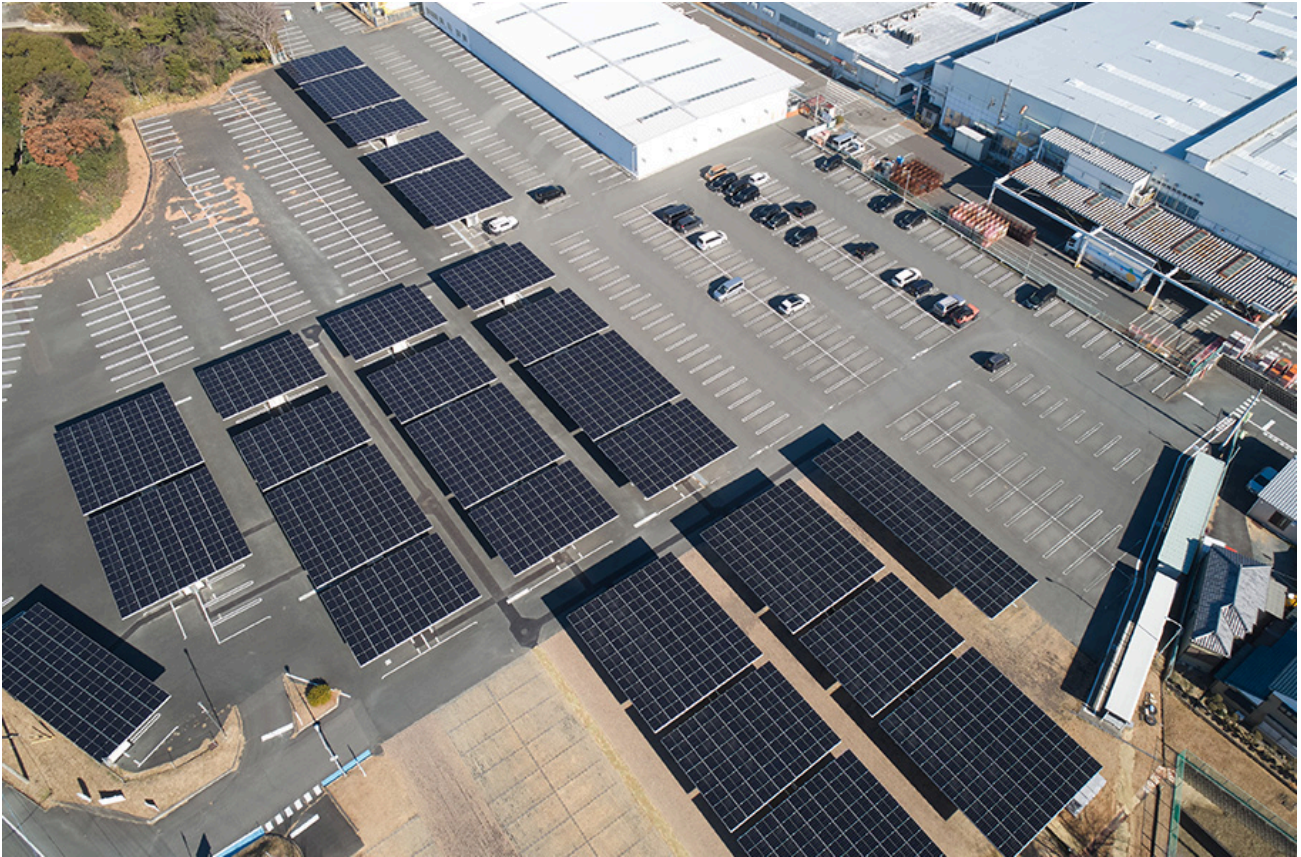
Carport solar power generation equipment newly installed in the employee parking lot
