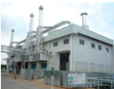
Gas engine generators at YMMWJ [Specifications] Gas engine generators Three generators with maximum output of 2,735kW [Steam used for] resin coating, metal coating, die casting [Reduction of CO 2 emissions by LPG fuel reductions] 400t-CO 2 /year * YMMWJ: PT. Yamaha Motor Manufacturing West Java
