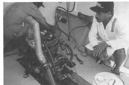
Staff work with engineers in the installment of an ME125E at a Suva boatbuilding factory.
