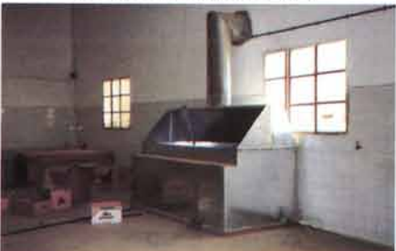
④ A new service shop, twice as wide as the current one.
