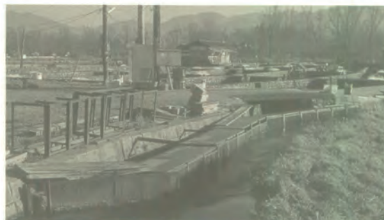
The entrance of the sluice leading to the ponds (in background) is covered with a fence for catching debris like floating sticks and leaves. To ensure a smooth flow of water the fence is extended for some distance.
