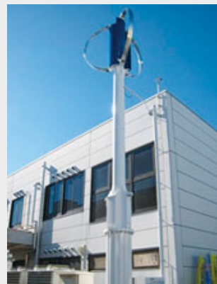
Vertical wind power generation system, which is quieter than the propeller type (Nakaze Factory)
