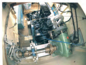
Engine room and power transmission mechanism (taken by using a wide-angle lens)
