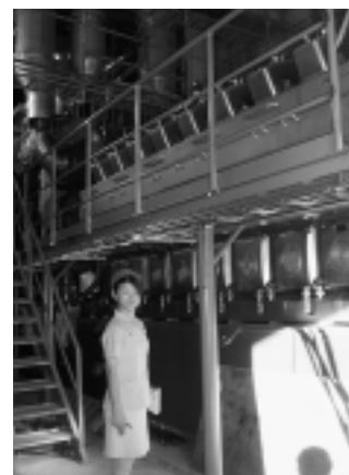
The generator installed at the headquarters factories is run by a V-18 engine with a displacement of 360 liters and cylinder bores of 30 cm. This generator supplies roughly half of the factories' electricity
