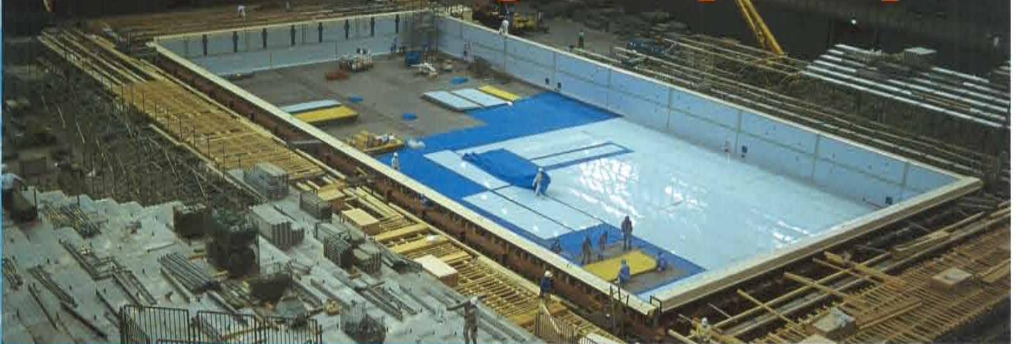
The assembly work proceeds at full speed to meet the opening of the World championship at Fukuoka
