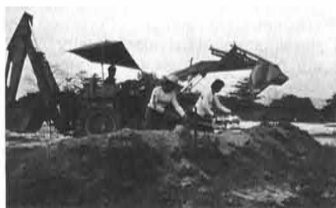
A bulldozer and shovel loader are used to make up a training course.
