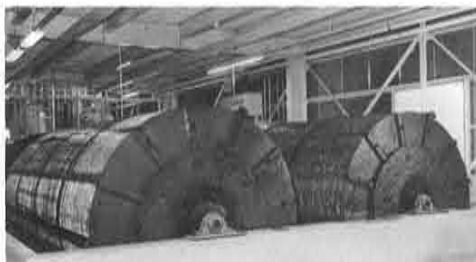
Water disposal equipment
